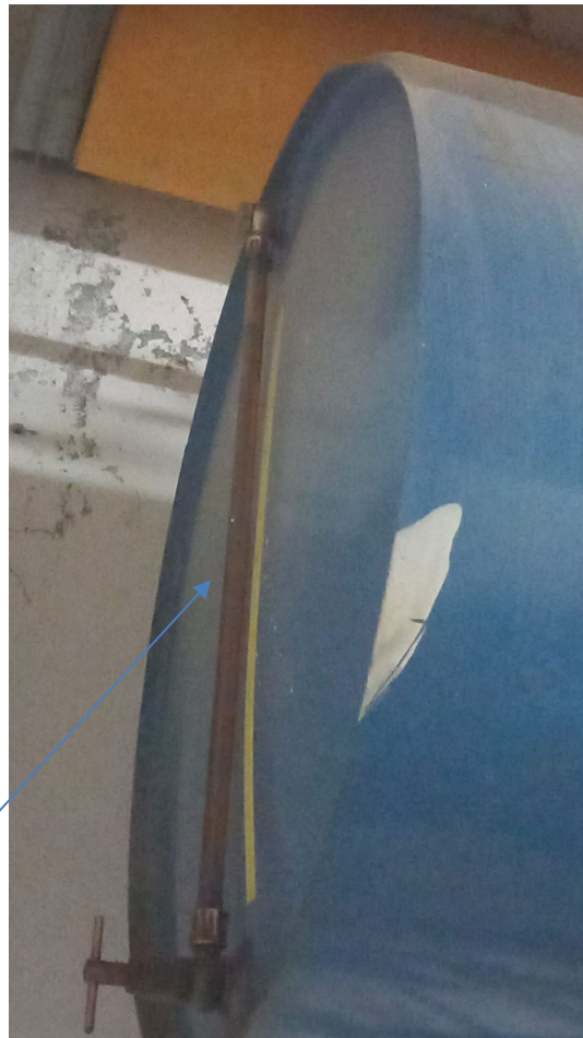
Sight glass for the fuel filling level (in the Diesel genset compartment)
